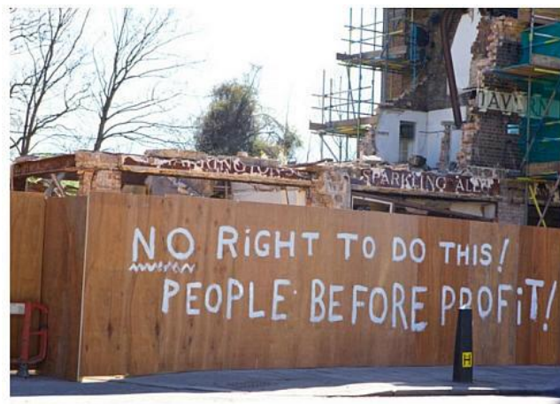
Councillors are consulting on what action to take after the Carlton Tavern was demolished
